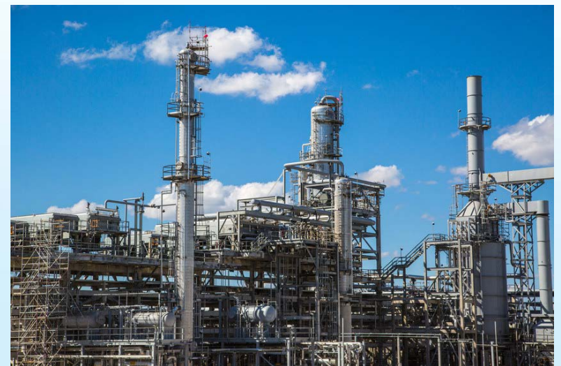
Buckeye Texas Partners condensate splitters
